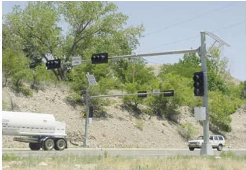
Three 3-section signal heads (solar powered). Lights are green until fire station activates.
